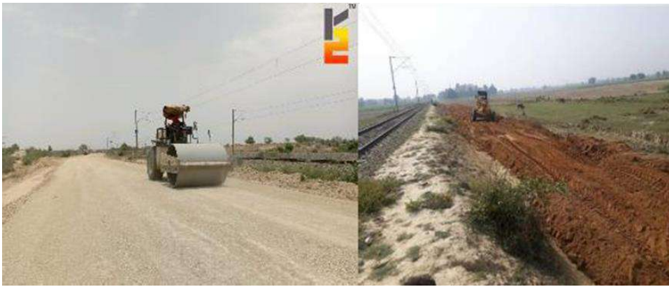
Vindhya Telelinks Limited Power Distribution Varanasi FY 2017-18
